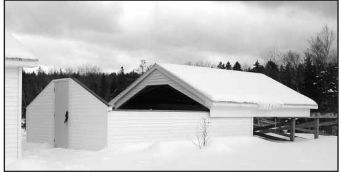
The roll-off with the roof partially open.
