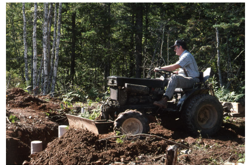
Walter Urban of Avonport volunteered his time and tractor to back-fill the foundation columns for the roll-off track. (Sept 24th 1996)
