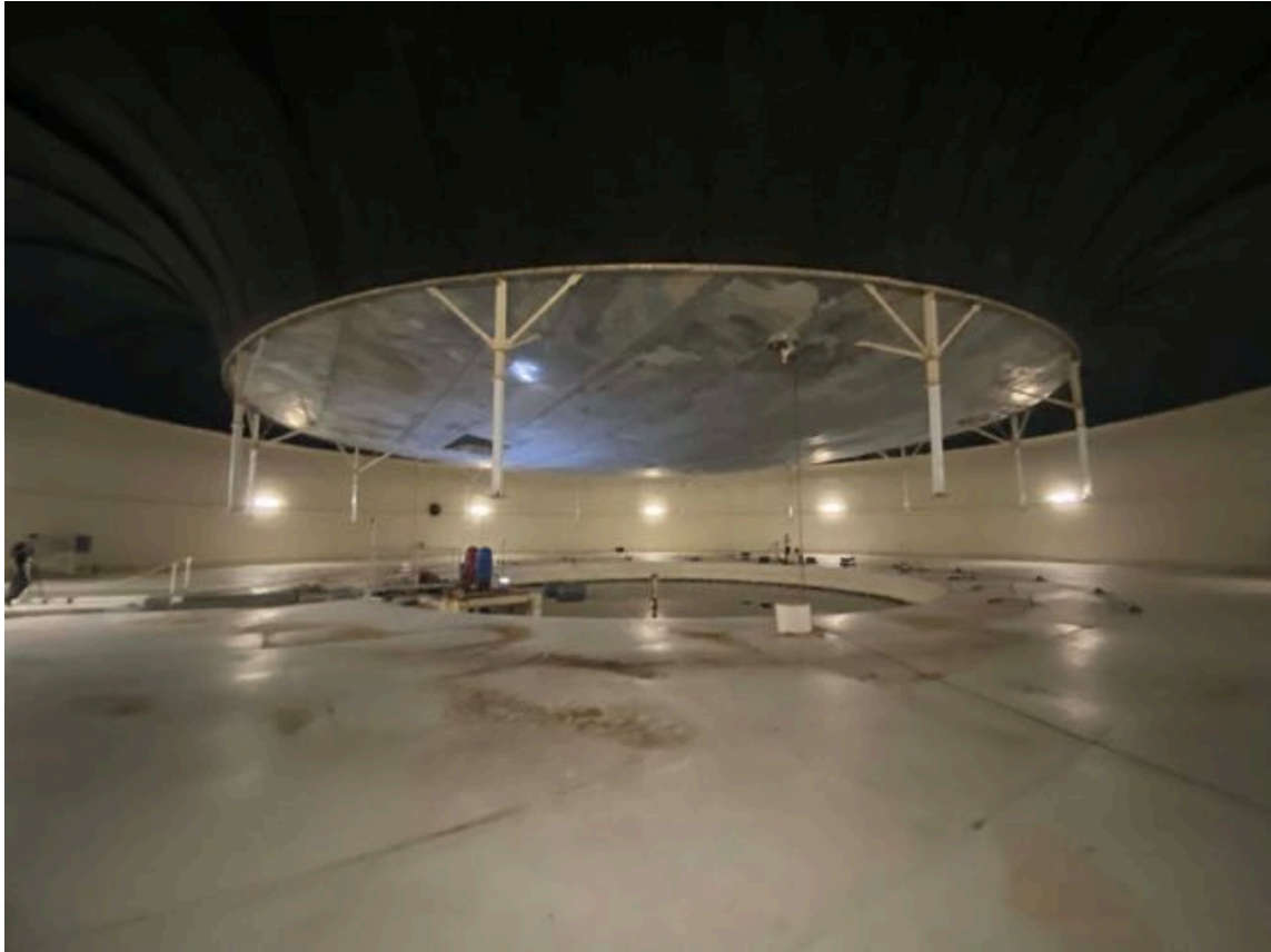
This is the lung that pressurizes the Biosphere. The biosphere is pressurized by the concrete weight suspended by a rubber bladder.
